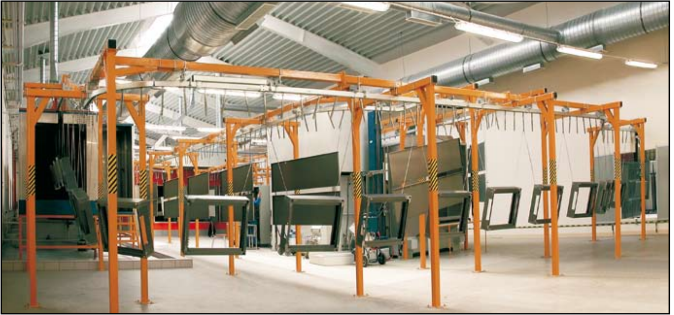
Automatic powder paint shop
