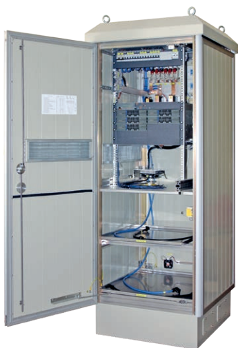
Outdoor telecommunication cabinet
