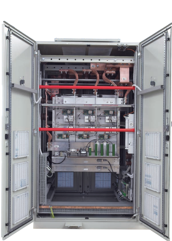
Excitation cabinet for 600 MW generator - rectifier box
