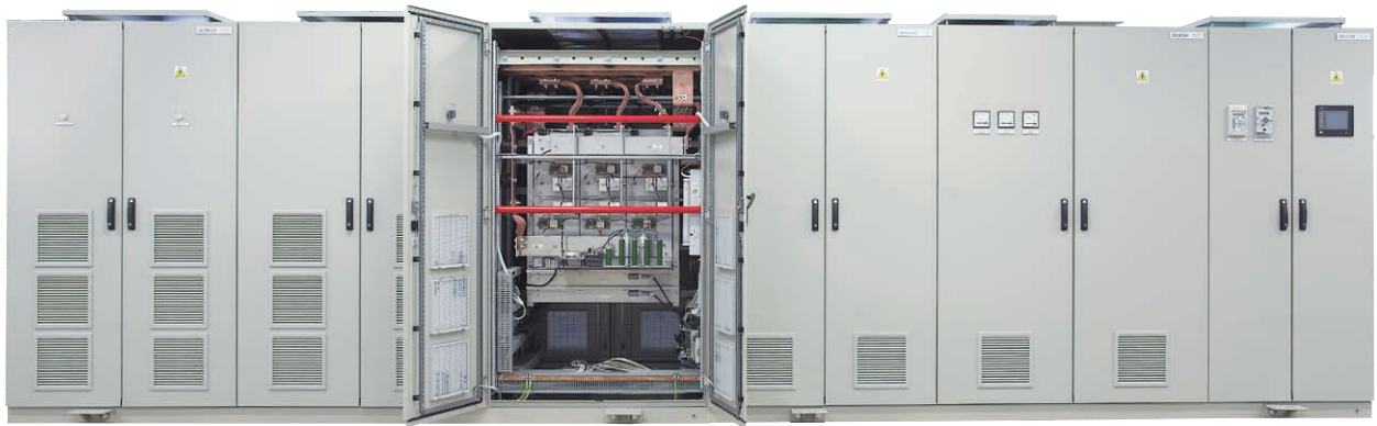
Excitation cabinet for 600 MW generator
