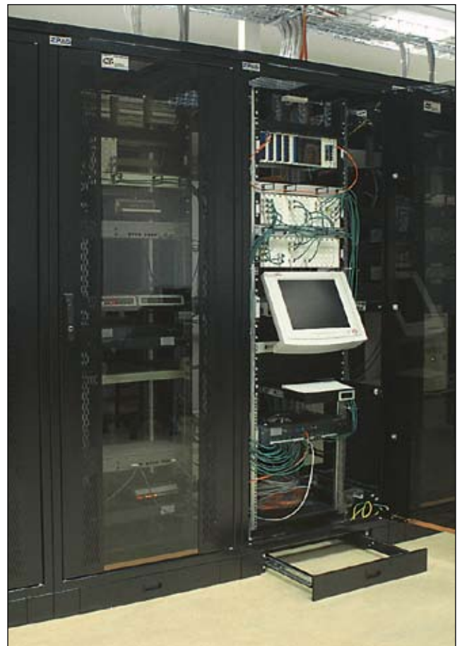
Server room equipped with SZB SE cabinets. Installation was performed by MCP Ltd. from Kraków, Poland ( http://www.mcp.pl )
