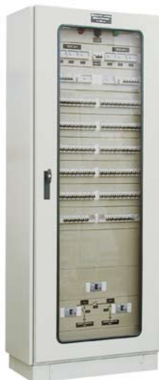
Double-section switchgear with modular equipment
