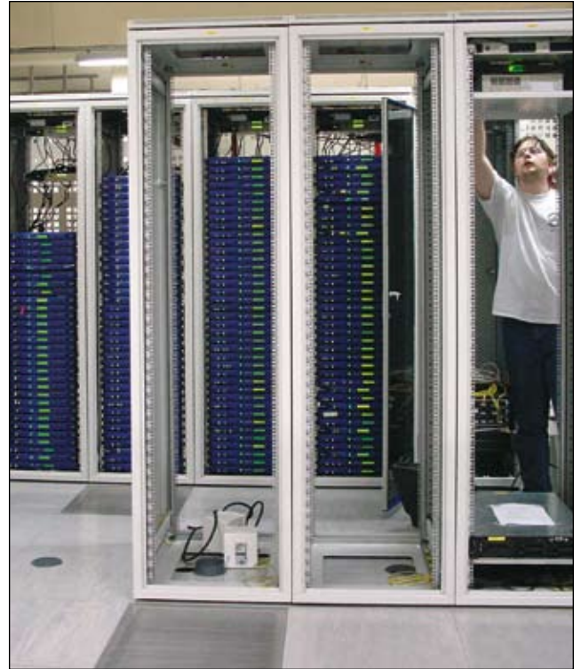
Installation of servers in SZB cabinets in OVH's internet server room in Paris
