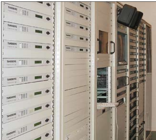
Stub-end station in the branch of Telefonía Polska - Zachód Sp. z o.o. in Stargard Szczeciński. Installation designed and manufactured using SZB cabinets, performed by VECTOR Sp. z o.o. from Gdynia (Poland) - http://www.vector.com.pl
