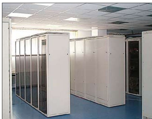
SZB cabinets installed in the headquarters of BPT "TELBANK" S.A. in Warsaw (Poland)
