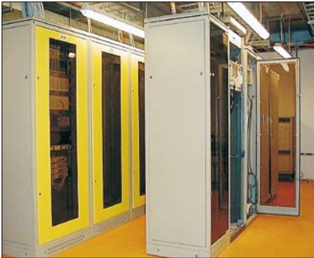
Main distribution room in the Stock Exchange Warsaw building. The whole system is designed and manufactured on the basis of SZB cabinets. Installation performed by ALMA S.A. from Poznań (Poland) - http://www.alma.biz.pl
