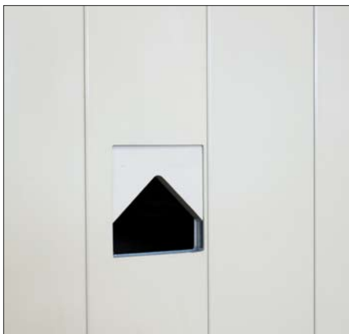
Cable entry - view from the outside of the cabinet
