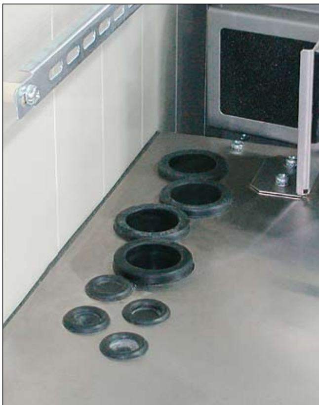
Cable entry made of rubber gland seals
